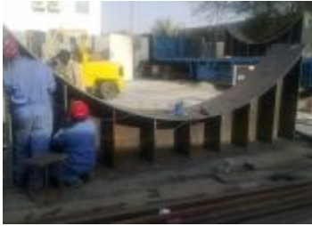
Saddles for large dia pipes
